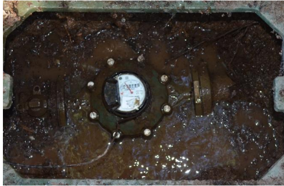
The above picture shows standing water inside of a meter box.
