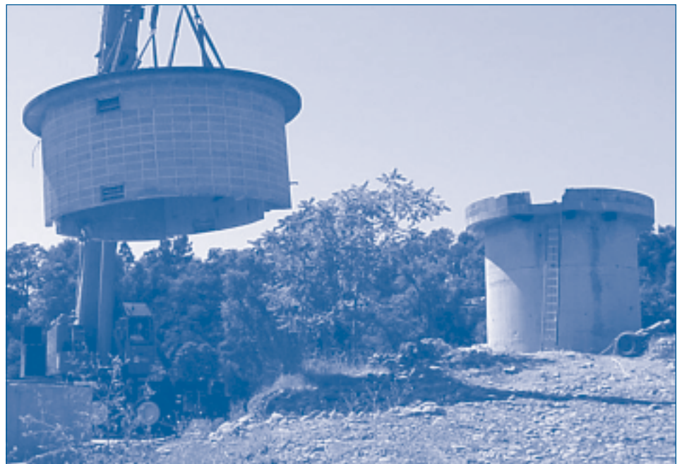
Once an important feature of the district's water production process, the tower portions of the Ranney collectors will no longer be necessary once the new treatment plant is complete.
