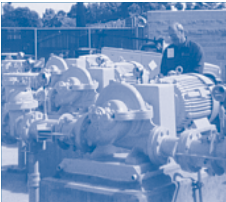
A new pump station, among other improvements, will ensure high quality water gets delivered to Carmichael Water District customers, even during an emergency.
