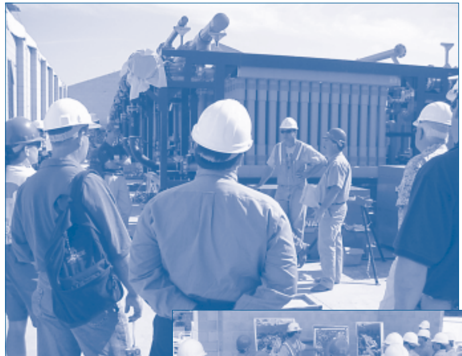
Visitors view the microfiltration units where water will be filtered by tiny hollow fibers. Each cylinder has 20,000 hollow fibers to filter out the smallest contaminants, ensuring the highest quality water for district customers.
