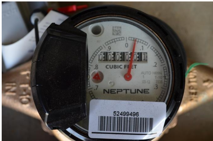
The above picture illustrates a typical water meter in Carmichael (notice the red triangle).
